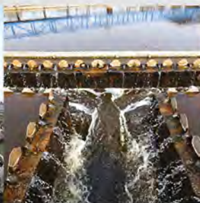
Waste Water Treatment Plant
